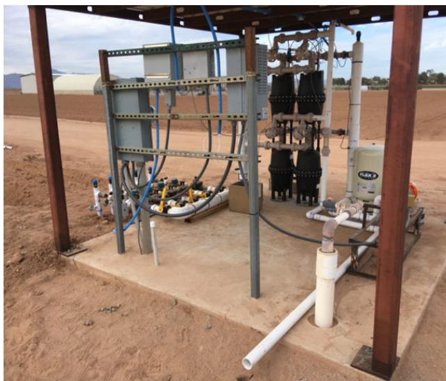
Photo 5. New irrigation pump station installed in Fall 2017, and used for irrigation experiments at Maricopa Agriculture Center.
